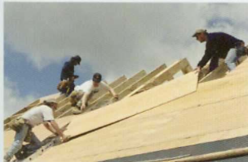
Sheathe trusses with plywood, but stagger the sheets to provide a strong roof surface.
