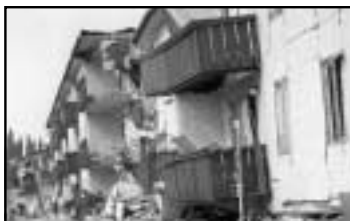
A collapsed apartment building in '94
