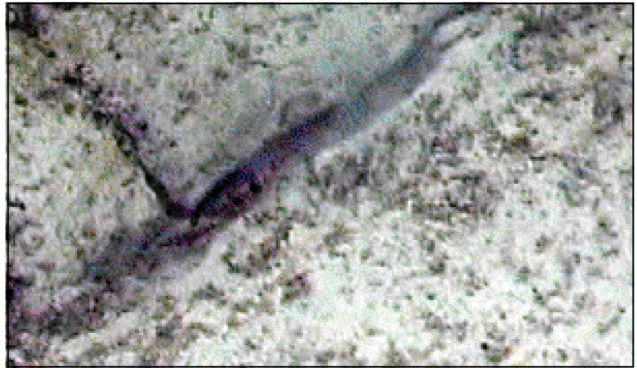
It took 20 minutes for the author to clear a 3-foot section of what initially appeared to be a crooked seam in the sandy area, but revealed was a straight, deep seam. (photo by Lora Little)
