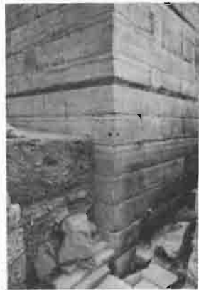
The huge retaining wall at the southwestern corner of the Temple Mount from the time of Herod the Great.
