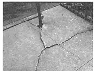
Sidewalk cracks display three-corner joints.
