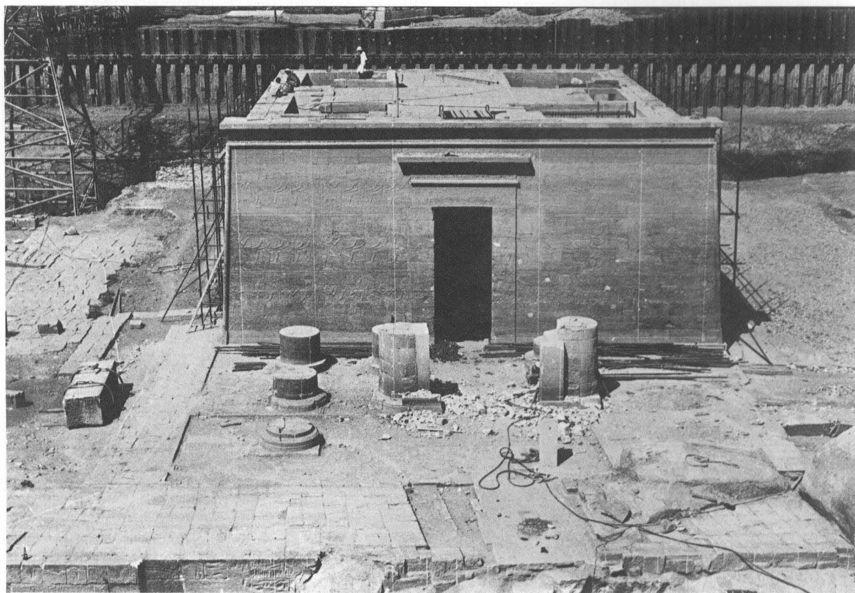
PLATE I. Temple of Isis built by Ptolemy II Philadelphus after removal of the Second Pylon and the Hypostyle Hall
