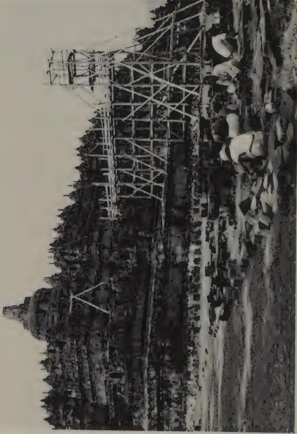
Restoration work in progress on the Borobudur Temple, Indonesia, 1969. An international campaign for the protection of Borobudur was officially launched with the signing of a formal agreement between the Indonesian government and UNESCO on January 9, 1973. UNESCO/Mireille Vautier.
