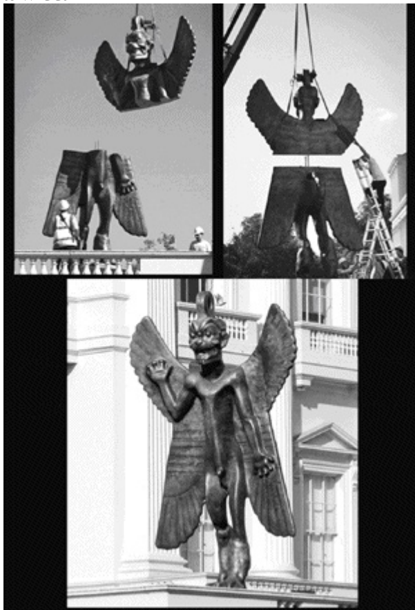
FIG. 86 – The statue of Pazuzu by Italian artist Roberto Cuoghi during and after installation on the “Nash House” in the road leading to Buckingham Palace, within the legendary area called The Mall.
