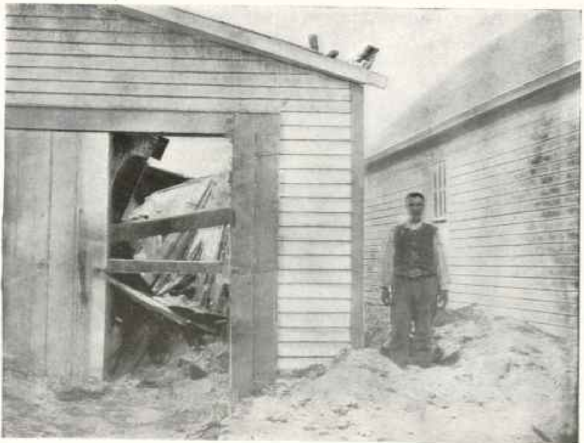
PHOTO BY W. J. KRUMHOLTZ SHOWING ROOF OF FISH HOUSE AT KADIAK BROKEN DOWN FROM WEIGHT OF ASHES, JUNE 14, 1912
