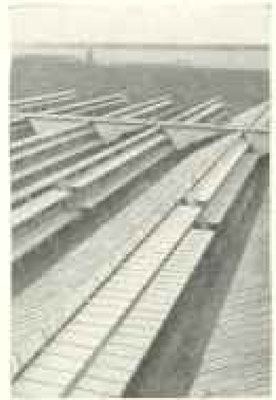
Example of air lock roof construction with Fenestra Continuous Center Pivoted Sash.
