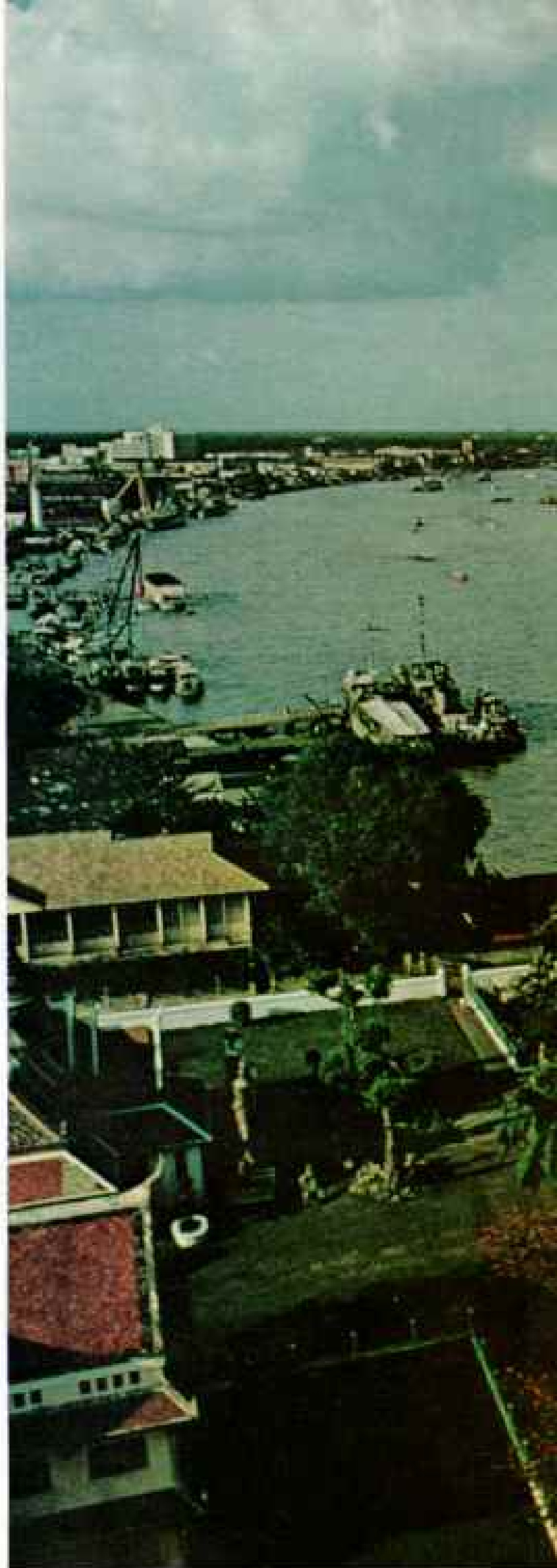
Angels in need of earthly help, statues atop Wat Arun receive a coat of epoxy resin to protect them from weather and disintegration. Traffic fumes, lightning, and the monsoon's wrath perennially besiege the famous Bangkok landmark, looming high on
