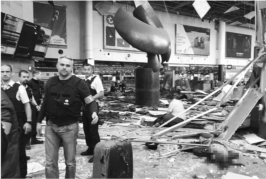
Figure: Ceiling tile collapse at Brussels departure lounge, showing undamaged walls and sculpture.
