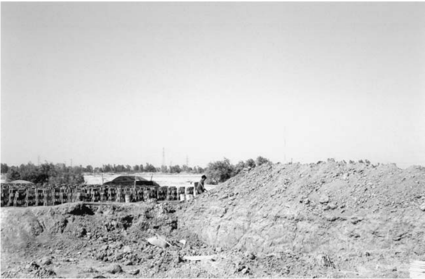
Plates 20 and 21. The new technology on the brickyards: a gasoline pump above; an earth excavated by an excavating machine below.
