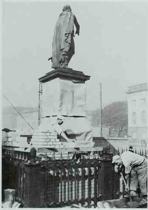
Two masons erect a sturdy cocoon of brick, mortar and heavy paper to shelter a statue in Berlin. Even neighborhood war memorials were bricked up for protection against bombs.
