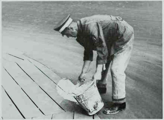
A workman paints a white circle on a wooden traffic island in Berlin. White markings on curbs and other obstacles helped citizens avoid them during blackouts.
