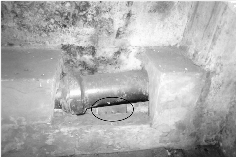
Photo 8: Delousing chamber at Stutthof, interior view, west wall; cast iron connection pipe to the oven located outside the delousing chamber and used to heat the air inside the chamber. The pipe was originally surrounded by masonry similar to that visible in the photograph, but of perforated brick. One of these bricks is still visible today, underneath and behind the pipe (circle). © Carlo Mattogno
