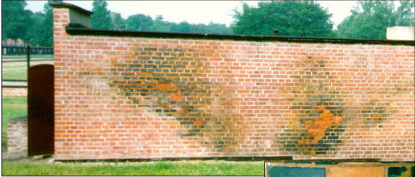
Photo 14: (top): delousing chamber in Stutthof, east side. The wall exhibits two large blue stains (iron cyanide), unequivocally proving the use of Zyklon B. © Carlo Mattogno
