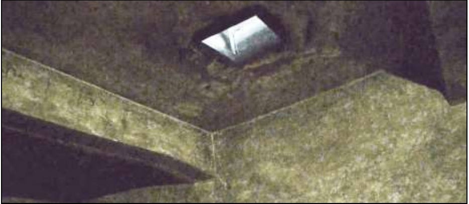
Figure 6: Photograph of hole near original dividing wall and door.
