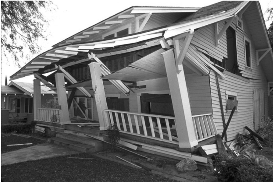
FIGURE 2-2 Northridge, California, earthquake, January 17, 1994. Buildings, cars, and personal property were destroyed when the earthquake struck. Approximately 114,000 residential and commercial structures were damaged, and 72 deaths were attributed to the earthquake. Damage costs were estimated at $25 billion. FEMA News Photo.
