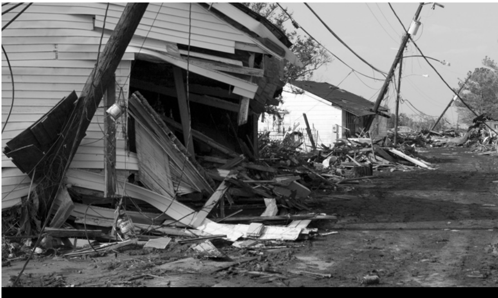
New Orleans, LA, September 18, 2005 Damage to homes and property in Lower 9th Ward due to Hurricane Katrina. Andrea Booher/FEMA
