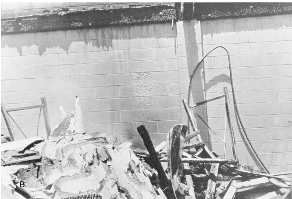
Figure 11.4 These photographs depict (A) chipping or splintering, commonly known as spalling, on a brick wall caused by a hot spot at the scene and (B) another example of spalling on a cinder block wall. ( Los Angeles County Sheriff's Department. )
