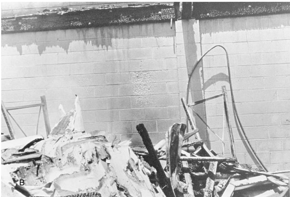
Figure 11.4 These photographs depict (A) chipping or splintering, commonly known as spalling, on a brick wall caused by a hot spot at the scene and (B) another example of spalling on a cinder block wall. ( Los Angeles County Sheriff's Department. )
