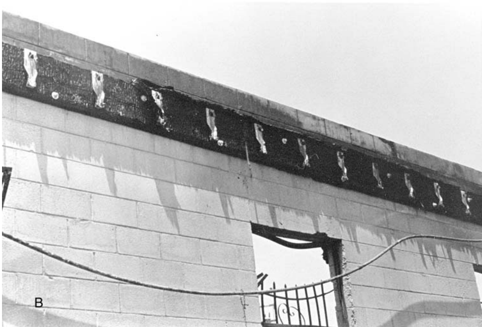
Figure 11.5 (A) Melted safety glass may indicate exposure to heat for a period of time, thereby suggesting a point of origin of the fire. (B) Deformed pipe as a result of the heat of the fire. (C) Typical appearance of burned lumber, referred to as “alligatoring,” indicating the surface texture of the burned wood. ( Los Angeles County Sheriff’s Department. )
