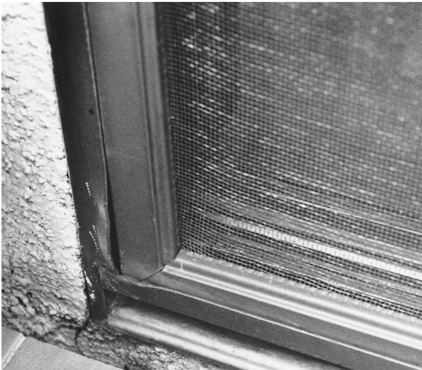
Figure 14.2 A window is often a point of entry in a case of breaking and entering or burglary. This screen shows prying marks in the lower left corner. ( Los Angeles County Sheriff's Department. )
