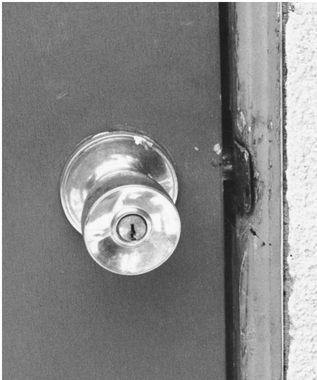
Figure 14.4 Exterior doors are another favorite point of entry. ( Los Angeles County Sheriff's Department. )
