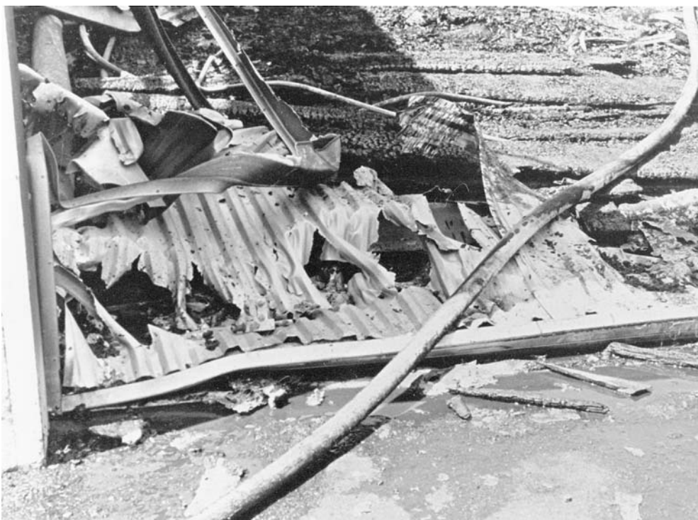
Figure 11.3 A melted aluminum awning indicates the approximate temperature of the fire. Aluminum melts at 660.2°C. ( Los Angeles County Sheriff's Department. )
