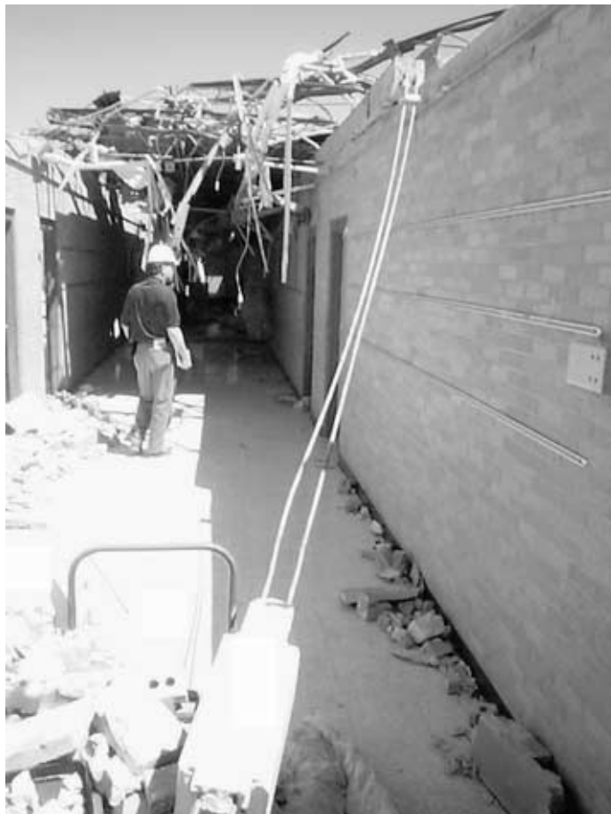
Figure 5-6 Failure in this load path occurred between the bond beam and the top of the unreinforced masonry wall. This school building was in the path of an F4 tornado vortex.
