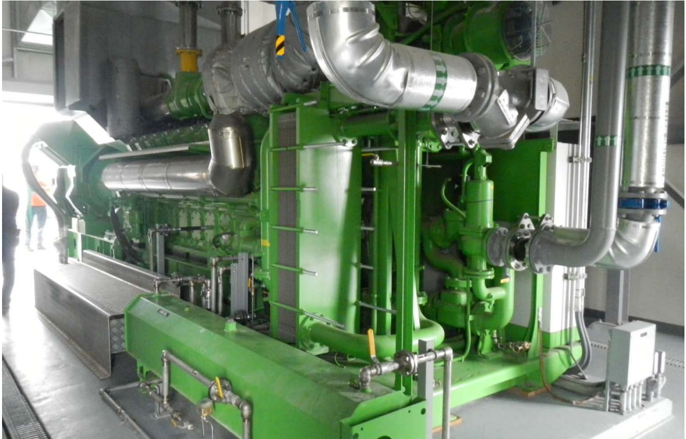
Butte County Landfill-Gas-to-Energy Project
