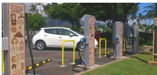
Figure 15 Fast charging station
