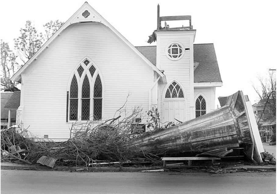
The Main Street United Methodist Church after the storm. Photograph by Joe Tomasovsky.
