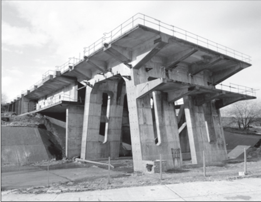
Figure 7.5. RAF Spadeadam, Cumbria, Blue Streak intermediate range ballistic missile test stand, 1959. Similar stands were built at Woomera, Australia for test launches. © Crown copyright NMR AA94/02010
