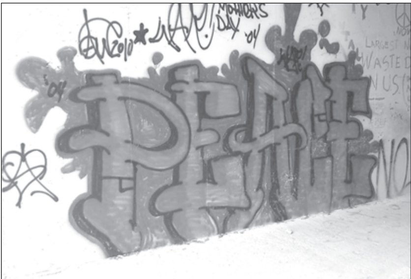
Figure 17.14. Graffiti in the tunnels.
