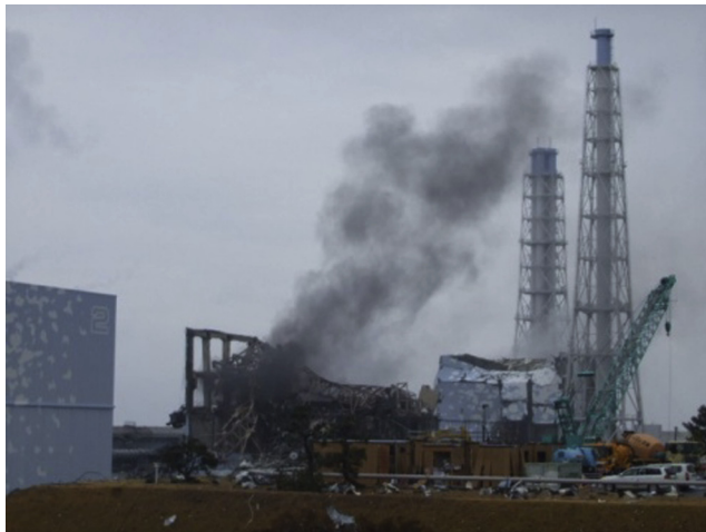
Figure 3.9 Damaged Unit 3 of the Fukushima Dai-ichi NPP after a hydrogen explosion on 21 March 2011 with emission of smoke. (Source: Reprinted with permission of TEPCO)
