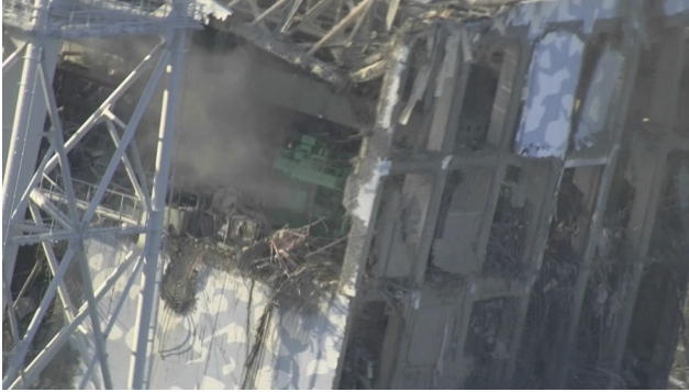
Figure 3.11 Damaged Unit 4 of the Fukushima Dai-ichi NPP after a hydrogen explosion on 16 March 2011. (Source: Reprinted with permission of TEPCO)
