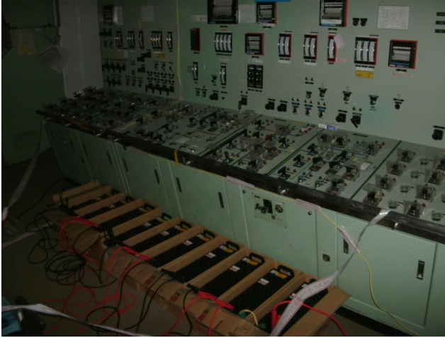
Figure 3.7 Reactor control room on 22 March 2011, with batteries supplying a power to run instruments in the control room. (Source: Reprinted with permission of TEPCO)
