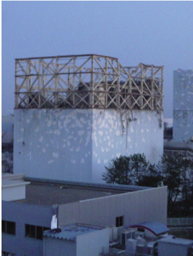
Figure 3.6 Damaged Unit 1 of the Fukushima Dai-ichi NPP after the hydrogen explosion on 12 March 2011. (Source: Reprinted with permission of TEPCO)
