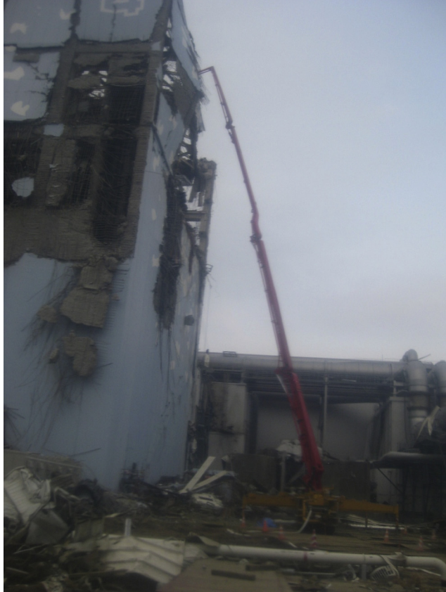
Figure 3.13 Unit 4 of the Fukushima Dai-ichi NPP on 11 September 2012. (Source: Reprinted with permission of TEPCO)
