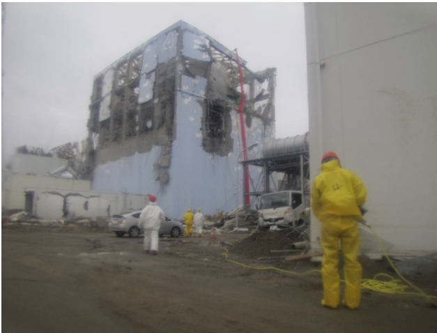
Figure 3.12 Damaged Unit 4 of the Fukushima Dai-ichi NPP after a hydrogen explosion on 22 March with water supply conducted by concrete pump truck. (Source: Reprinted with permission of TEPCO)
