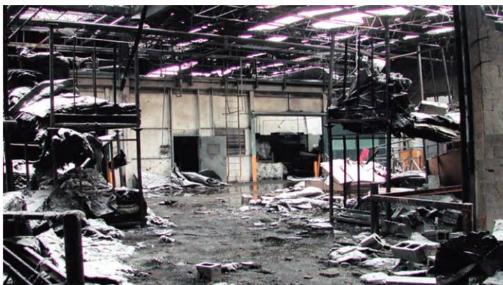
FIGURE 3.1 The aftermath of a dust explosion. Photo credit: U.S. Chemical Safety and Hazard Investigation Board (2006). Investigation Report: Combustible Dust Hazard Study, Report No. 2006-H-1.
