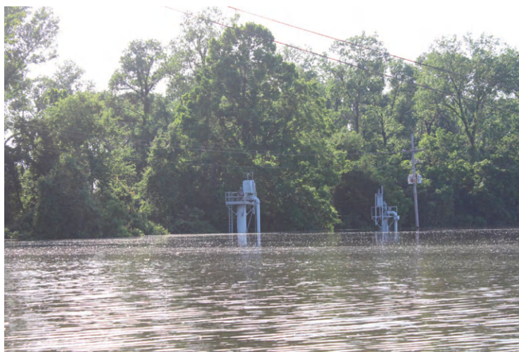
FIGURE 5.2 Electric powered water pumps are in danger of submergence and shutdown the rising Mississippi River in Vicksburg, Mississippi on May 6, 2011. Photo by H. Greenblatt. Source: Federal Emergency Management Administration, 2011.
