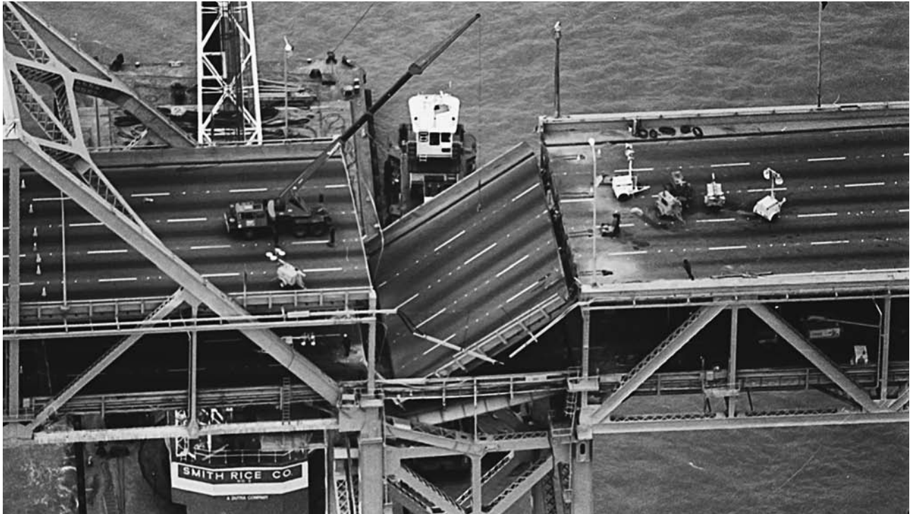
A crane mounted on a barge begins repair on the upper deck of the San Francisco–Oakland Bay Bridge, damaged by the Loma Prieta earthquake of 1989. ( Associated Press )
