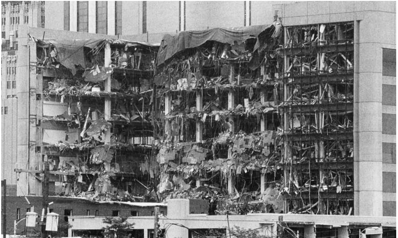
The Alfred P. Murrah Federal Building in Oklahoma City lay in ruins after terrorists exploded a truck bomb on April 19, 1995. (New York Public Library)
