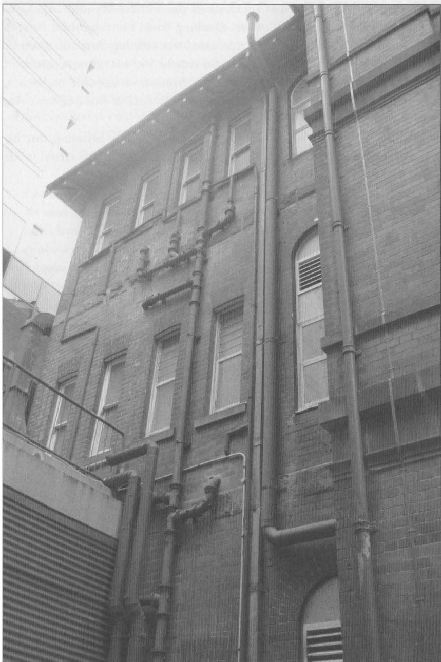
The Wall from which Andrew Williams Fell.
