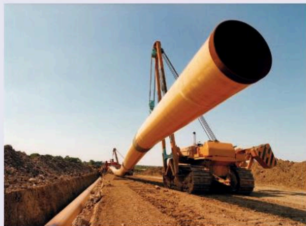
Fig. 11.8 An oil pipeline
