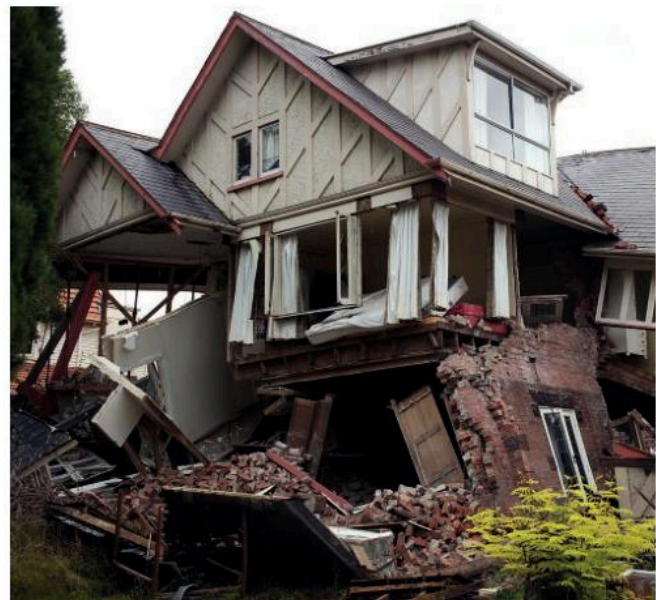
Fig. 3.9 The 2011 earthquake in Christchurch, New Zealand, brought down many buildings and killed 65 people
