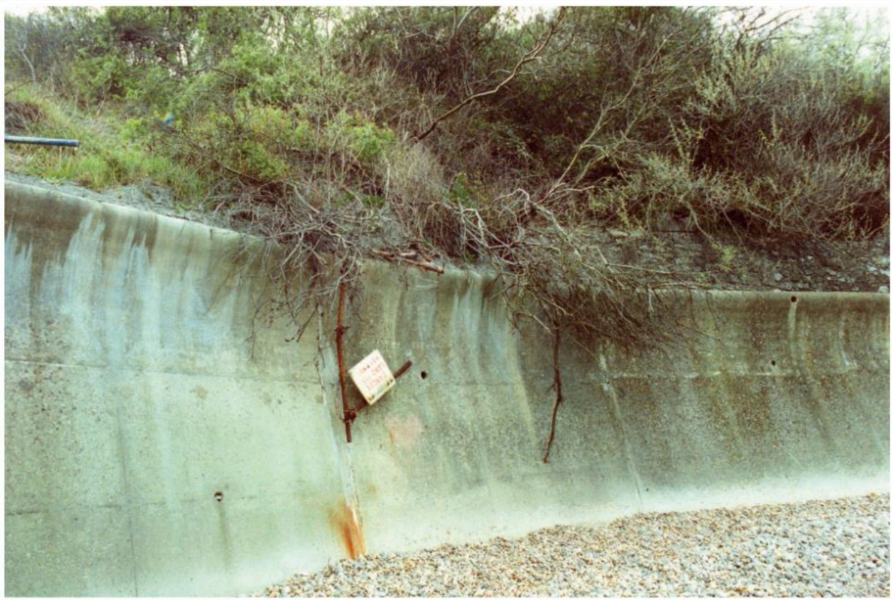
Fig. 5.29 A concrete sea wall at the head of a shingle beach with an unstable cliff behind it. The sea wall's purpose is to deflect waves, so its top is curved outwards.
