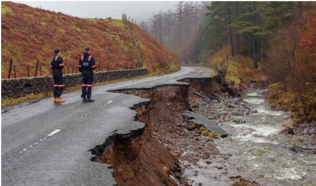
Fig. 4.31 The A591 main road through Cumbria collapsed and washed away, December 2015
