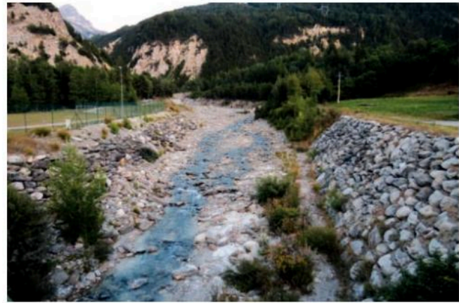
Fig. 4.25 Reinforced riverbanks at Bramans in the French Alps. Snow melt in spring causes increased discharge, making the river very powerful.
