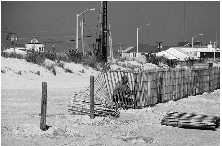
Fences are installed along the Manasquan, New Jersey, beach to reduce the transport of windblown sand. Keeping sand on the beach instead of having it blow away inland provides a measure of storm protection. (Photograph courtesy of MACGES.)
