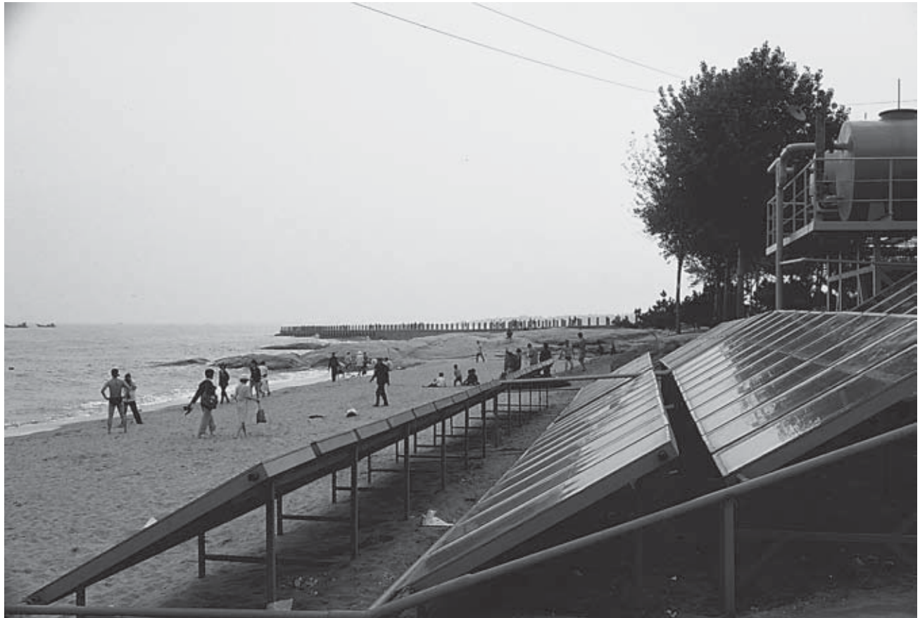
Solar collection panels at Beidaihe. China is now making an effort to move toward more renewable energy resources, such as solar power. PHOTO BY JOAN LEBOLD COHEN.
