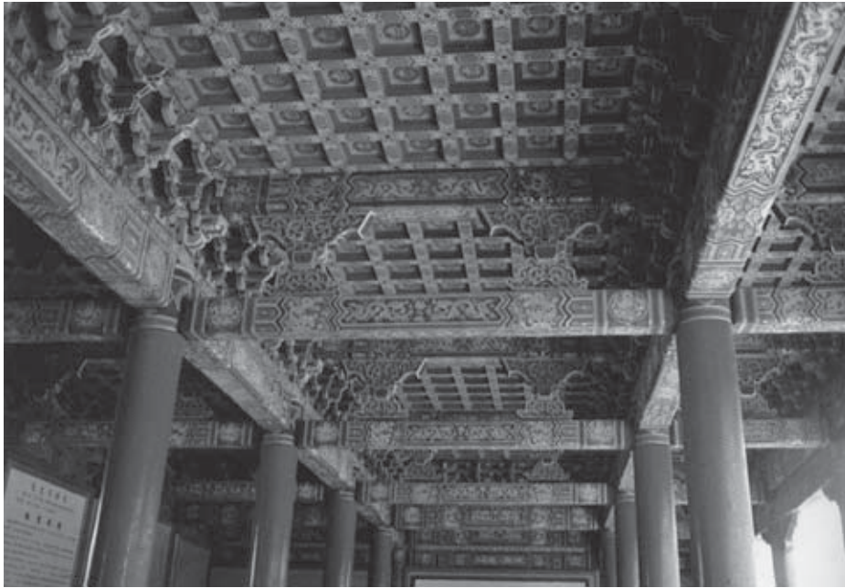
Detail of the wooden ceiling of the Hall of Eminent Favors. The ceiling, like those in the Imperial Palace, is coffered and brightly painted. Golden dragons writhe within the coffers and on the cross beams. PHOTO BY JOAN LEBOLD COHEN.
