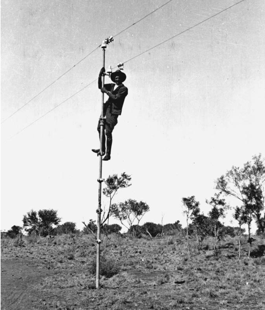
Frequent repairs to the line were made by operators resident in the many telegraph stations located all across central Australia. Bob Carew is working on this line in 1921. (Image courtesy of the State Library of South Australia, SLA: PRG1365/1/133)
