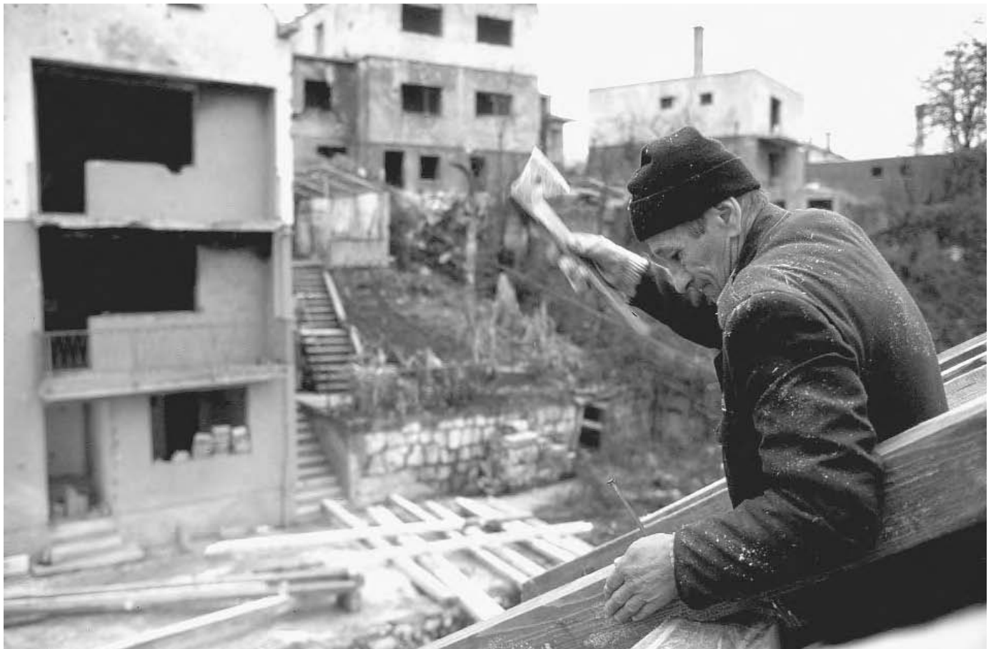
Reconstructing Bosnia-Herzegovina one nail at a time. A man puts a new roof on his war-damaged home in the Brbavica district of Sarajevo, 1997. (Getty Images)
