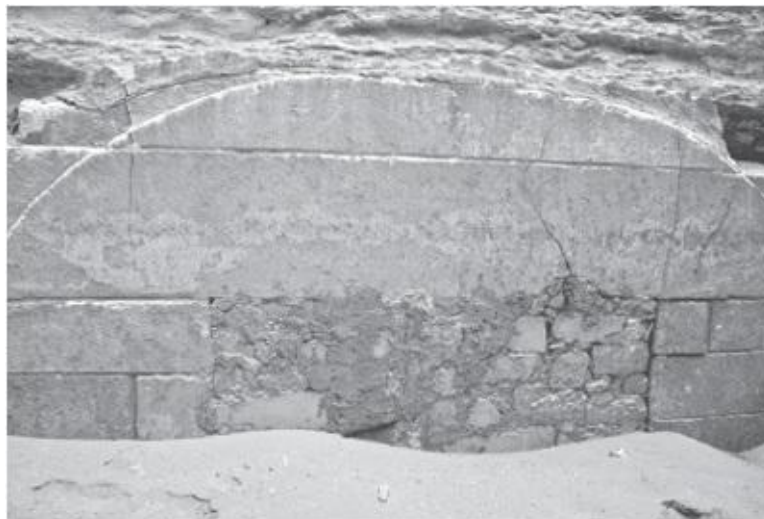
Figure 14.9. Another blocked-up entrance with an electric wire at the bottom
