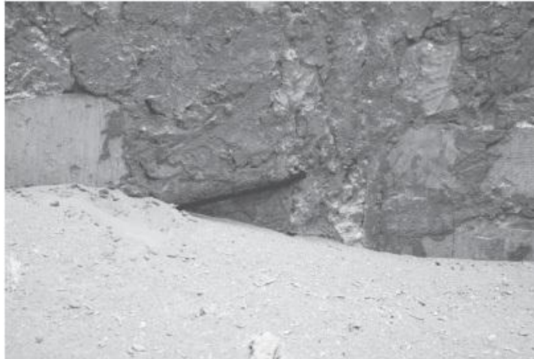
Figure 14.10. Close-up of the black electric wire
