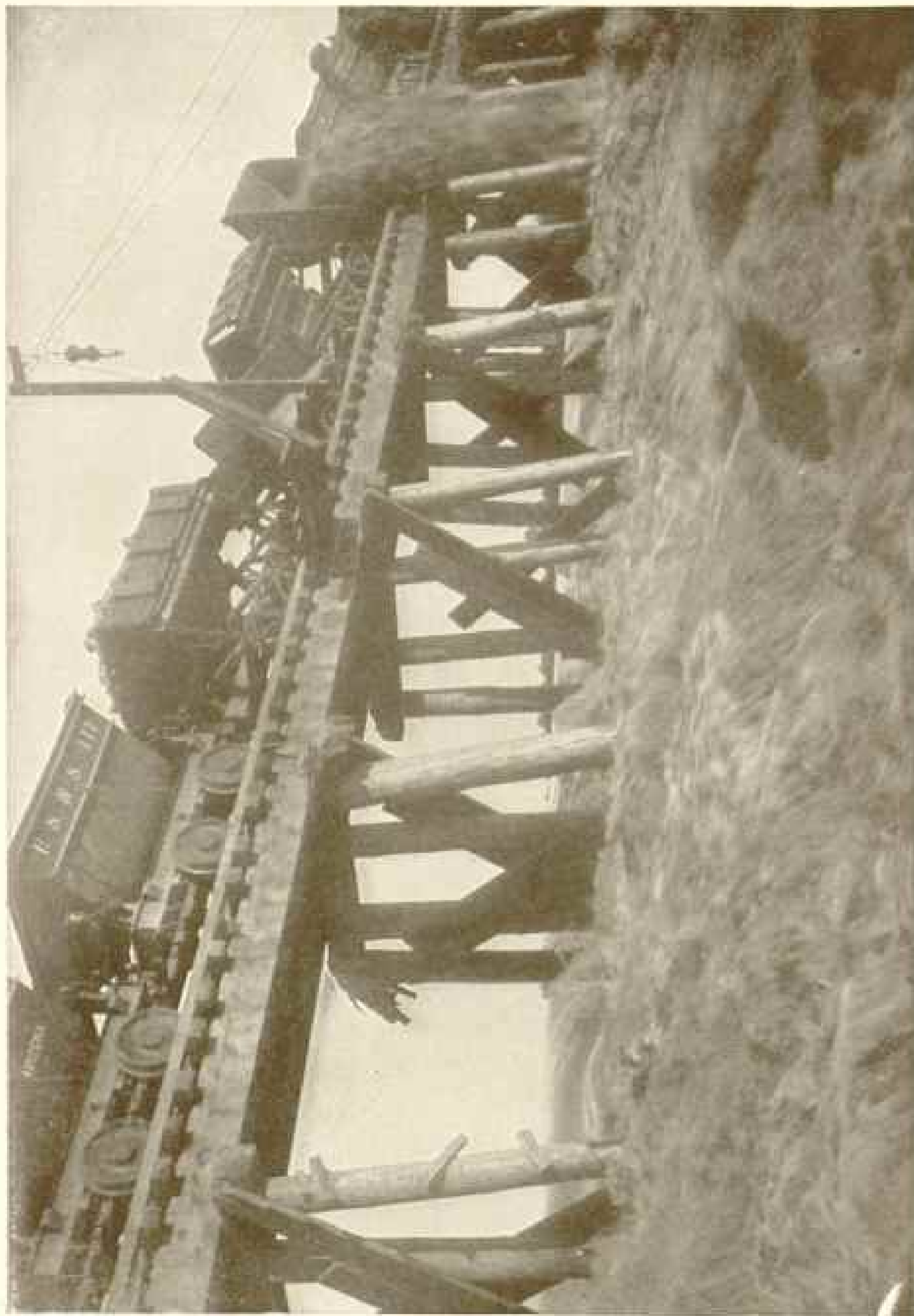
CLOSING COLORADO RIVER DURING CONSTRUCTION OF LAGUNA DAM, YUMA PROJECT, ARIZONA-CALIFORNIA Nearly 72,000 cubic yards of material were dumped into the stream before the closure was effected. The Laguna dam now completed is 4,280 feet long, 19 feet high, and weighs 600,000 tons
