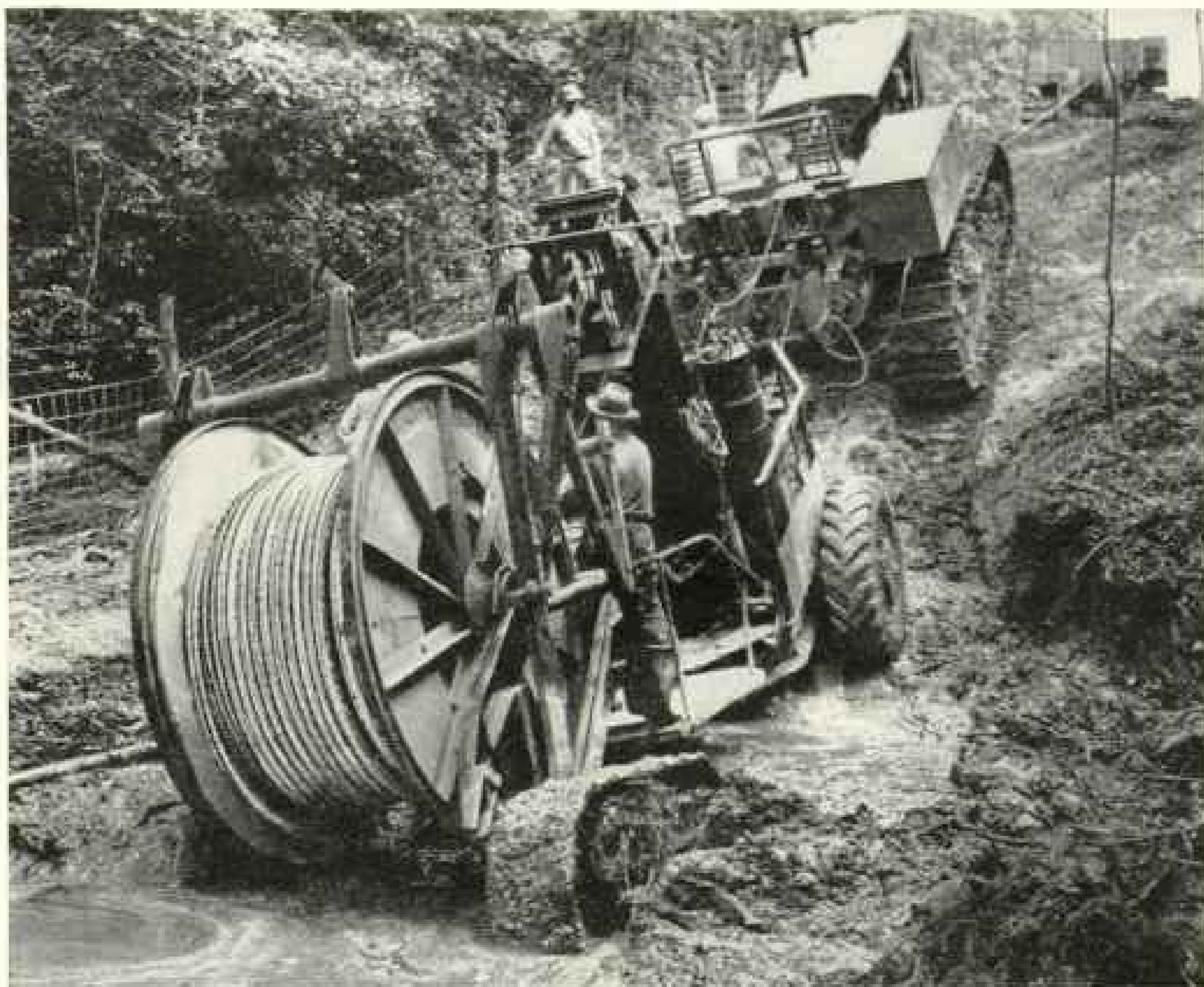
THIS LOOKS LIKE A WAR PICTURE but it's right here in the U.S.A. It shows a part of a telephone cable-laying job. We're planning to install 2,100,000 miles of Long Distance circuits within a year.
