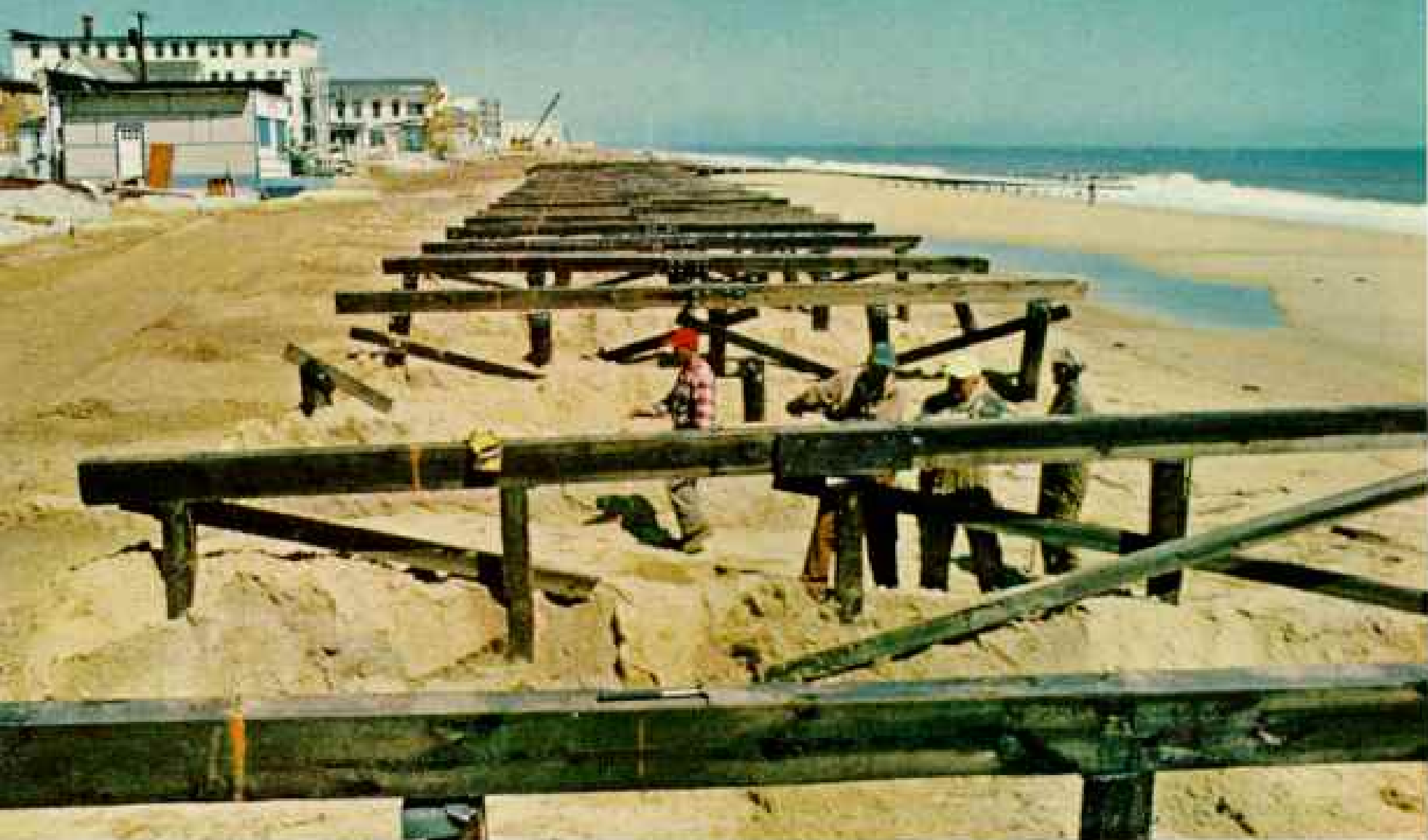
Battered boardwalk takes shape again at Rehoboth Beach, Delaware. Pilings and a few cross timbers weathered the storm, but planks washed away. Seaside cottages and motels were shattered.
