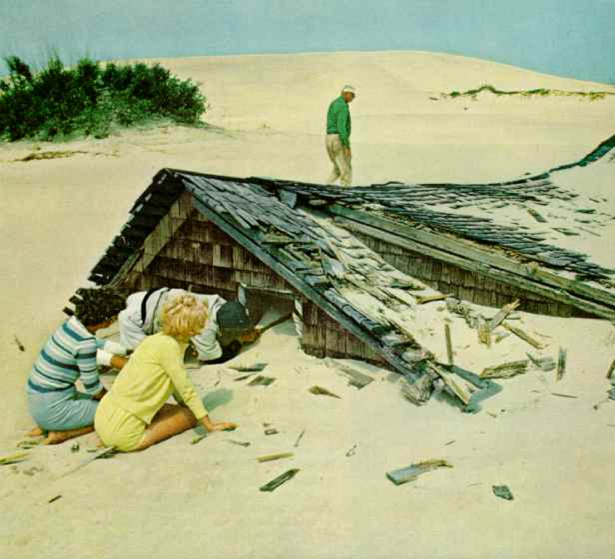
Buried to the eaves, this beachside house once sheltered a fisherman's family. Creeping inland, the sea of sand engulfed the village of Wash Woods, North Carolina.
