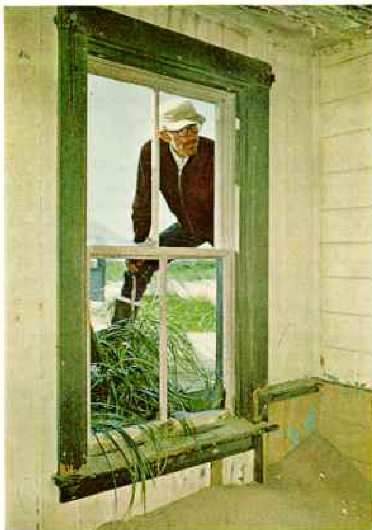
Slender fingers of marram grass creep inside a window of the long-vacant superintendent's house in 1964. Sand sifts in through every opening; drifts build in corners. No longer do brave men dash from its rooms to risk their lives saving those wrecked upon the island's shores while their wives stand at the windows "to watch the foaming white mountains of surf," as Mrs. Boutilier wrote to Mrs. Bell.
