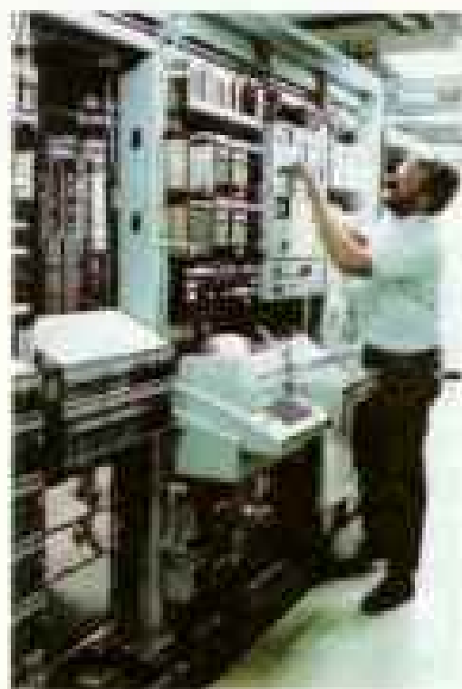
Roy Roman is the Bell System man in charge of Sedona's electronic switching system.
