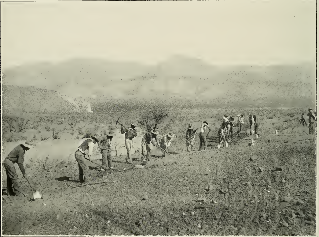
Indians (Apaches), survivors of Geronimo's Band, building a Road to the Roosevelt Dam, Arizona. (See page 89)
