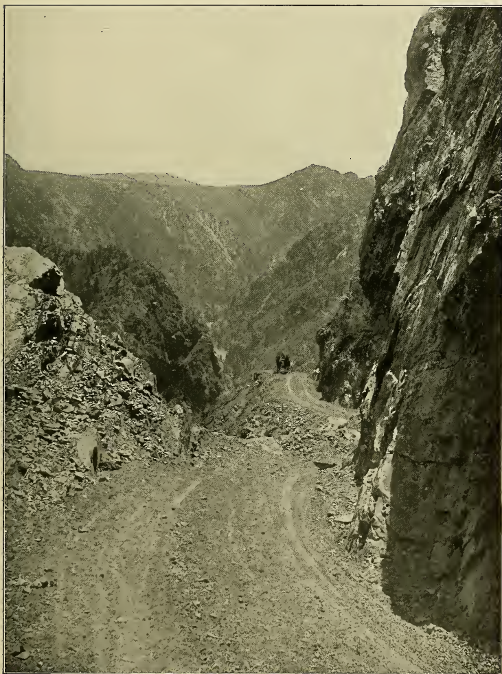
The Newly Constructed Government Road Up the Gunnison Canyon The road in places has grades out of the canyon of 24 per cent (see page 234)
