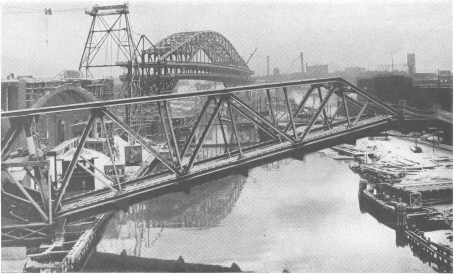
A LABYRINTH OF BRIDGES ACROSS CUYAHOGA RIVER, CLEVELAND, OHIO, INCLUDING THE NEW HIGH-LEVEL BRIDGE IN COURSE OF CONSTRUCTION
