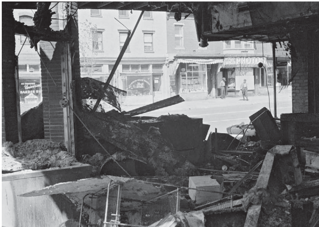
Building in Washington, D.C., destroyed during the riots that followed the assassination of Martin Luther King, Jr., April 1968. Library of Congress, Washington, D.C. (digital file no. 03132u)
