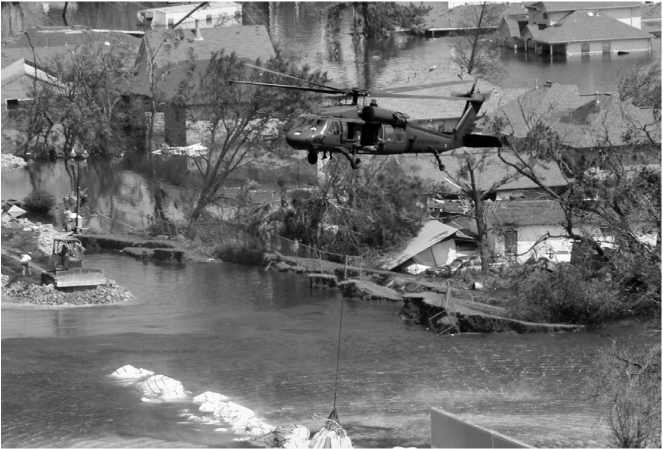
A National Guard helicopter works to repair a broken levy in New Orleans in this photo taken not long after Hurricane Katrina devastated the city.
