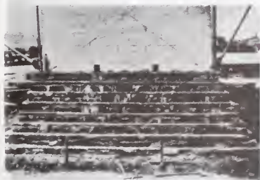
Thirty-six feet beneath the surface, the new foundation weighed 37,000 tons and covered more than three times the previous area.
