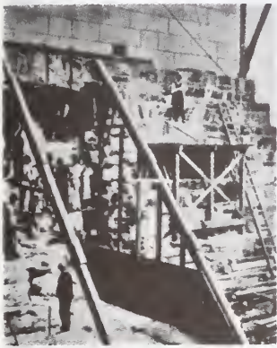
First, the center section of each side was removed and replaced by fresh concrete.
