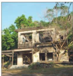
Charred remains of a once splendid Colonial villa, Kep
