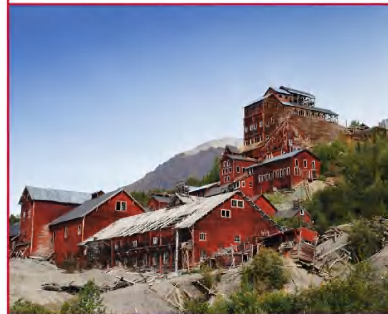
The 14-storey wooden mill stands almost as it did when the town was populated
