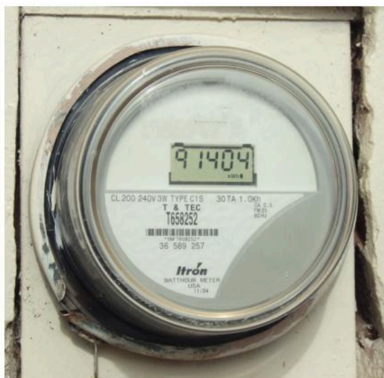
▲ Figure 11.6.1 Reading a digital electricity meter
