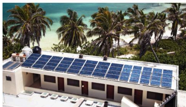
▲ Figure 9.1.5 An array of solar panels
