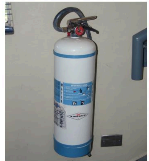
▲ Figure 11.10.2 Water fire extinguishers cannot be used on all fires
