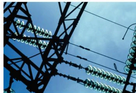
▲ Figure 11.1.2 Electricity cables and insulators on a pylon
