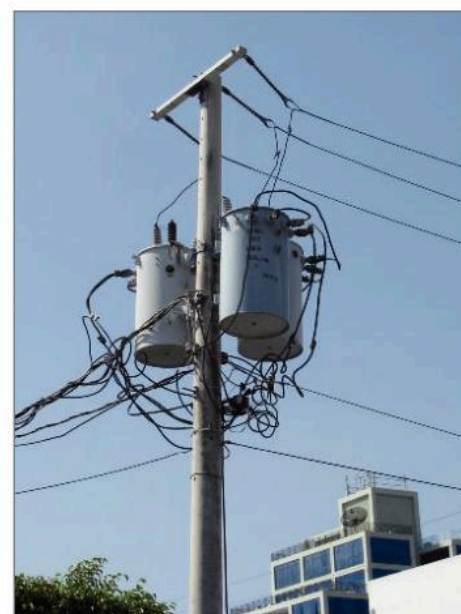
A telegraph pole with a transformer, bringing the electricity supply to a home
