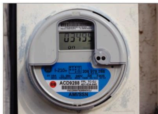
A digital electricity meter
