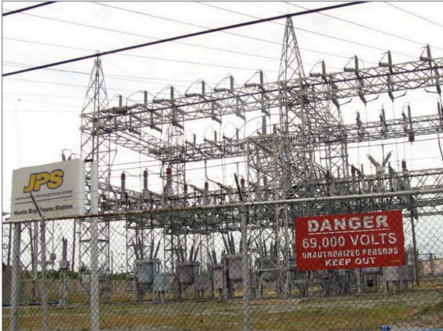
1 Hunts Bay Power Station. Electricity is transferred in the wires at a high voltage.
