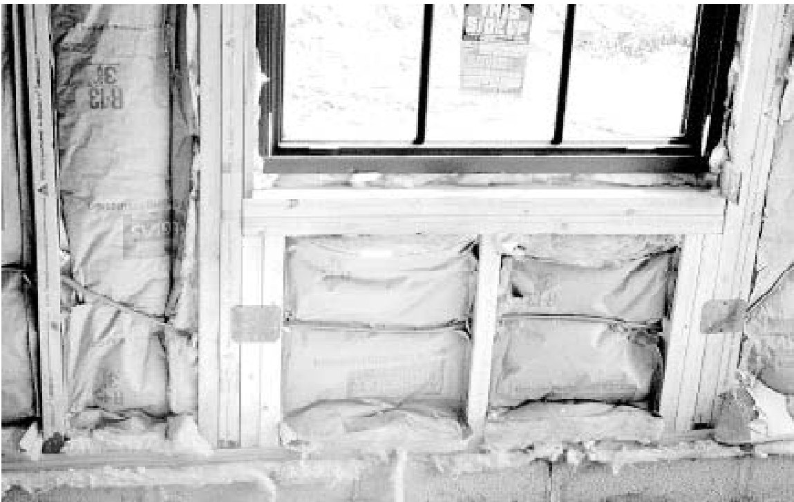
Fig. 1 What is wrong in this picture? The batt thickness is appropriate for the stud widths. However, the insulation is stuffed far inside the cavity, reducing its thickness and creating a large convection path in front. The kraft paper vapor barrier is not effective, because the paper is not joined at the edges. The method of installing the electrical wiring force the insulation installer to stuff the insulation behind the wiring. Fiber insulation is used instead of proper caulking around the window, and under the sole plate. Anything else?
