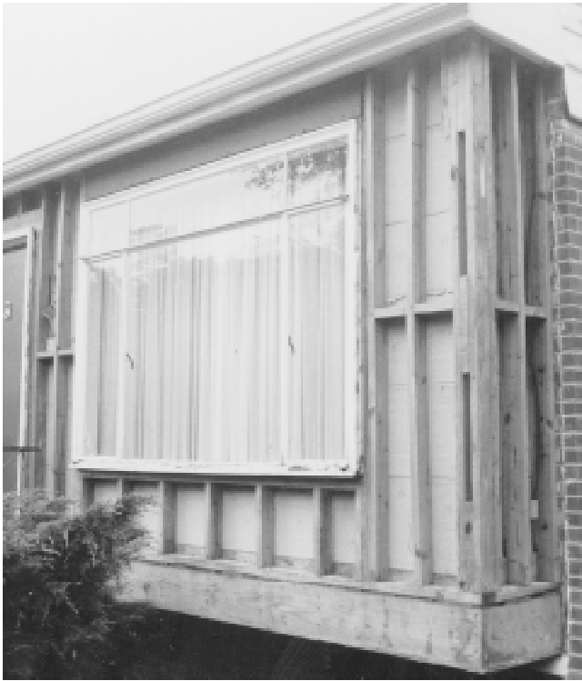
Fig. 4 Retrofitting stud wall insulation from the outside, first step The exterior siding and sheathing are removed. Porch light wiring penetrations in the wall are sealed.
