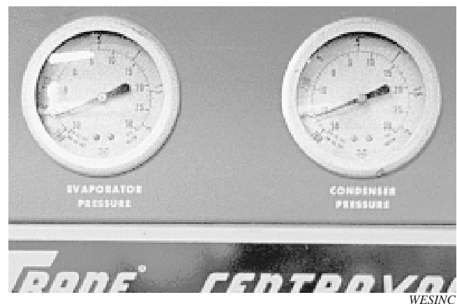
Fig. 2 Evaporator and condenser gauges These tell you immediately whether the machine has the minimum amount of refrigerant for efficient operation. They do not tell you the actual amount. The condenser pressure provides an uncertain indication of excessive charge.
