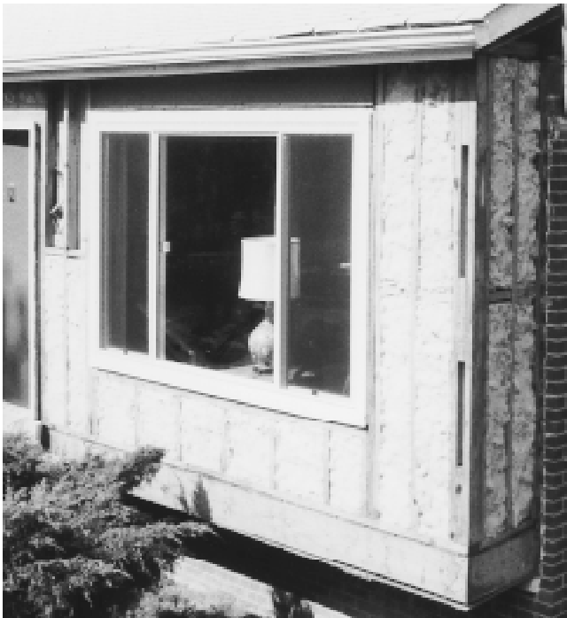
Fig. 5 Second step The old single-glazed window is replaced with a new double-glazed window. The stud wall cavities are entirely filled with insulation, being careful to leave no voids.
