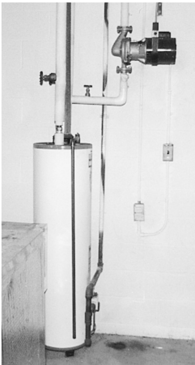
Fig. 1 Little water heater, big recirculation pump This pump is probably much larger than needed, although it is still only a fraction of a horsepower. Note that the hot water distribution and recirculation lines are insulated.
