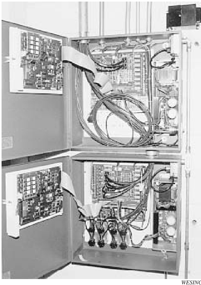
Fig. 5 Can you tell what this does? Neither can the maintenance staff. This is a local panel of an EMCS. It is much more difficult to understand than the facility's primary equipment. The EMCS requires its own specialized skills and additional manpower. Without these, the EMCS will fail and be abandoned.
