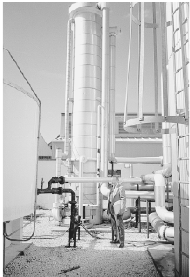
Fig. 17 Separated ice slurry system equipment The tall tower in the center is the evaporator. The ice storage tank is on the right. The chiller condensing unit is on the left.
