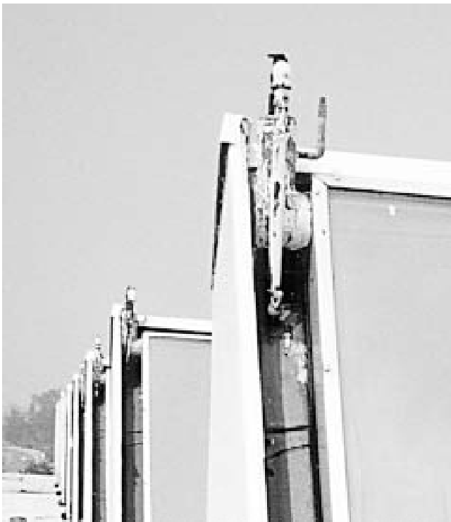
Fig. 3 Pressure relief valves to protect against stagnation This abandoned solar heating system failed to provide adequate protection against stagnation. The pressure became high enough to repeatedly vent the liquid, which contained antifreeze. The replacement water did not contain antifreeze. Eventually, the system was destroyed by freeze damage.
