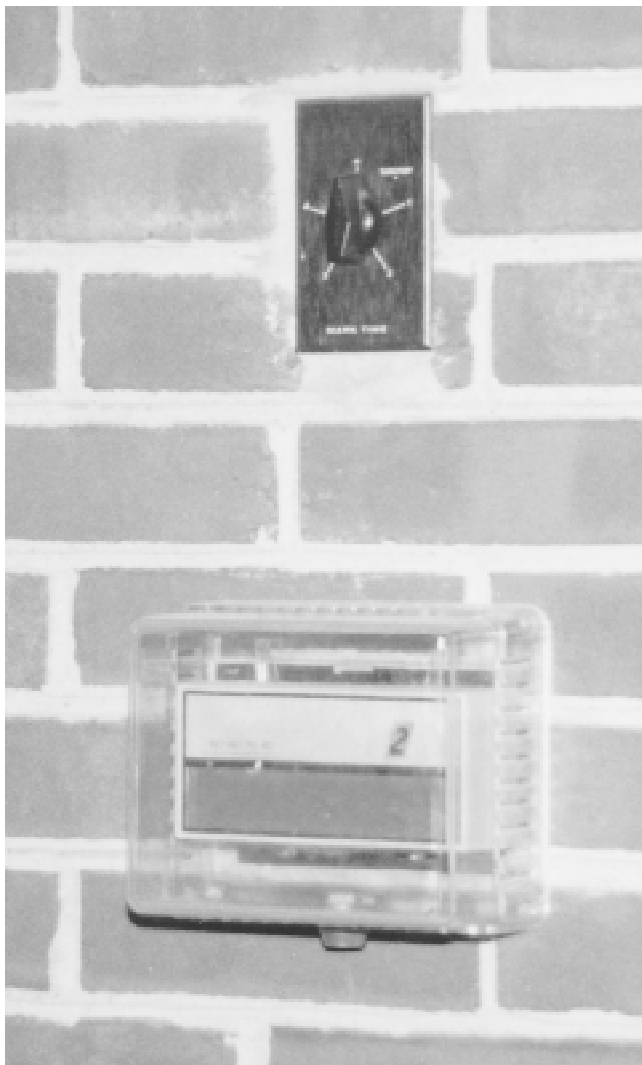
Fig. 1 Rundown timer used to control conditioning in a library function room This is very effective for the purpose. The space has no exterior exposure, so warm-up time is minimal. However, there is no placard to tell unfamiliar users what the timer does, or how to use it. Also, the locked cover on the thermostat is a bad idea.
