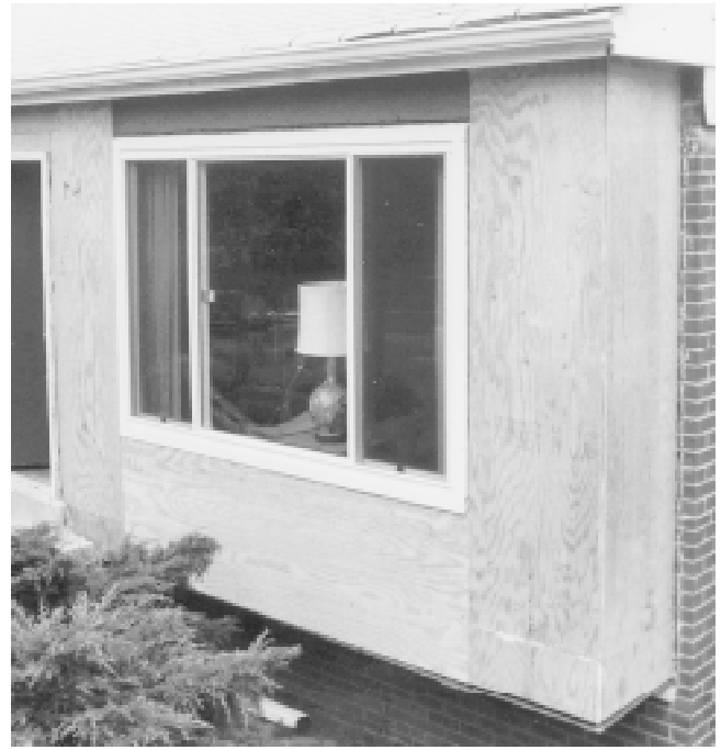
Fig. 6 Third step Strong exterior sheathing is installed, each panel caulked and nailed to the studs. This method of installation does not allow a satisfactory vapor barrier to be installed inside the wall, so impermeable paint is applied inside the house.
