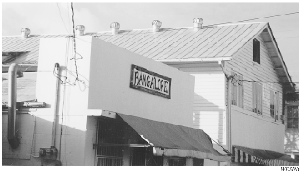
Fig. 4 Turbine ventilators These are well placed. Static ventilators would probably be as effective. A continuous ridge vent would be even more effective, more attractive, and less expensive. The gable end louvers are large, and could be even larger.
