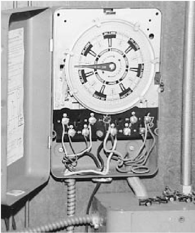
Fig. 5 The fate of any timeclock that lacks an effective override This old timeclock has been sabotaged in the usual way, by removing the “off” trippers, which are lying below the timeclock. An electronic timeclock without an easily accessible override would probably have been put out of commission in a more destructive way.
