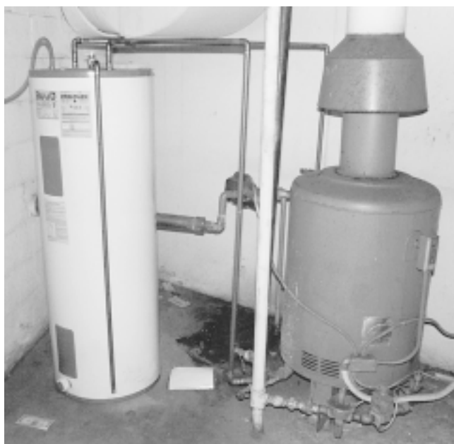
Fig. 1 Going the wrong way This old gas water heater in a government building was replaced with an electric heater, even though gas is much less expensive than electricity in this location.
