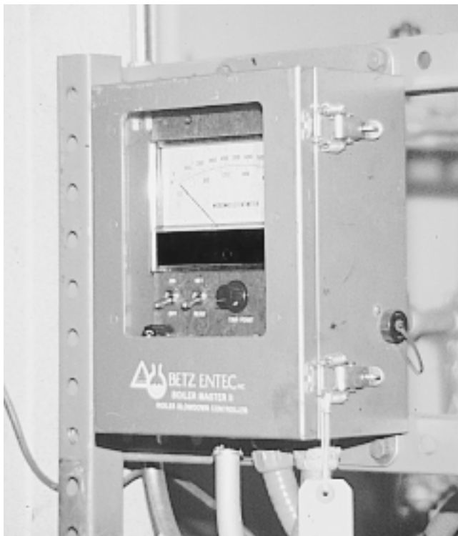
Fig. 1 Automatic blowdown controller The controller senses boiler water conductivity to activate surface blowdown.
