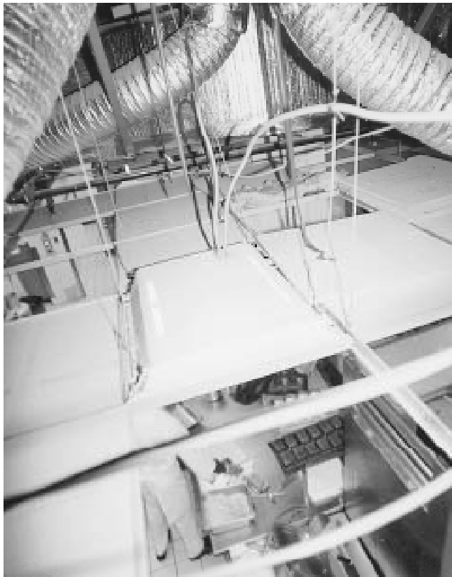
Fig. 1 Why grid-mounted light fixtures cannot be located efficiently The grid pattern limits the fixture location to increments of spacing that are too large for efficient placement. Also, duct and pipe installed above the grid may make it difficult or impossible to move the fixtures.
