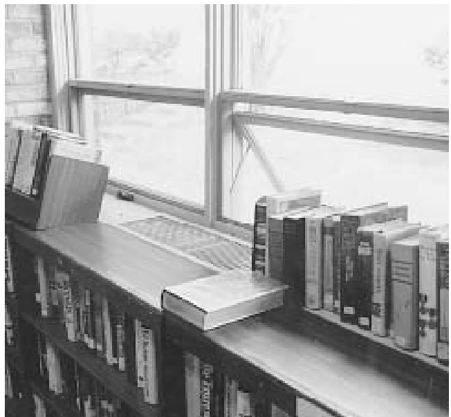
Fig. 2 Discharge to an open window Much of the heating or cooling energy goes directly outdoors through this library window. And, books may block the discharge to the space. Another case where the architect did not talk to the engineer. There are several possible solutions.
