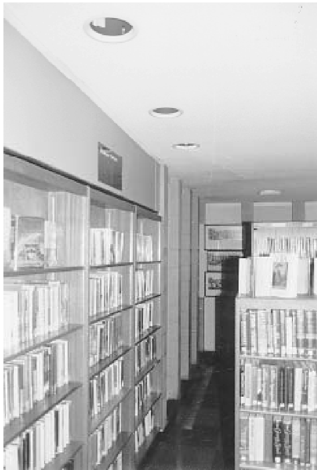
Fig. 1 Wrong fixtures for the application The dark interiors of these deeply recessed downlights absorb most of the light of the lamps. The light that escapes from the fixtures mostly goes into the carpet. Single-tube fluorescent fixtures, mounted on the ceiling surface, would require only a few percent of the energy of these fixtures, for a given amount of illumination on the books.
