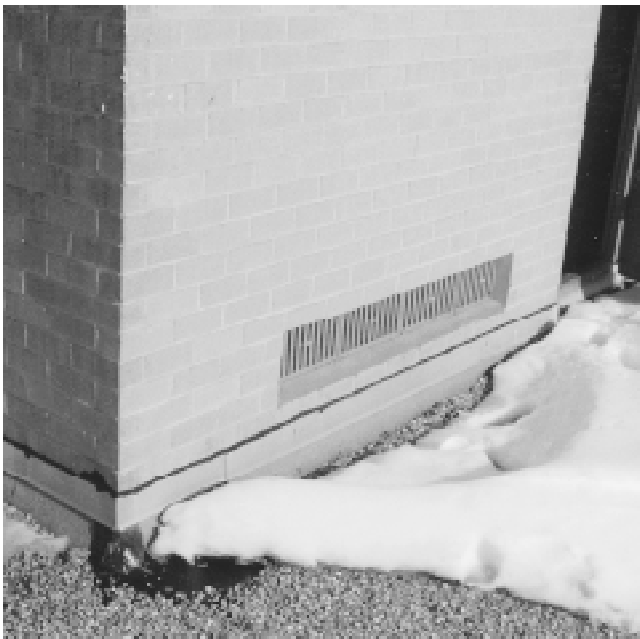
Fig. 1 Elevator shaft ventilation The melting snow shows that a lot of heat is being lost from this elevator shaft, which has a number of vents this size.
