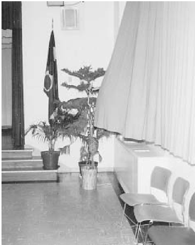
Fig. 1 Discharge trapped by drapery Almost all the heating output of this unit is discharged between the drapery and a large window. Much of the heat is lost by conduction through the window, and the small insulating value of the drapery is lost.
