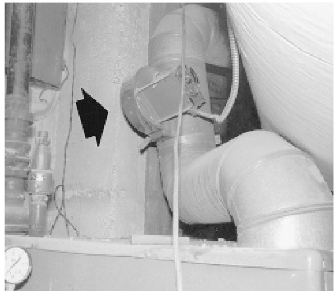
Fig. 2 Stack draft inducer This retrofitted unit, intended to solve a draft problem, was found running continuously. It should be controlled to turn off when the boiler is not firing. Otherwise, it increases standby losses and cools the flue, which kills the draft and causes flue corrosion.
