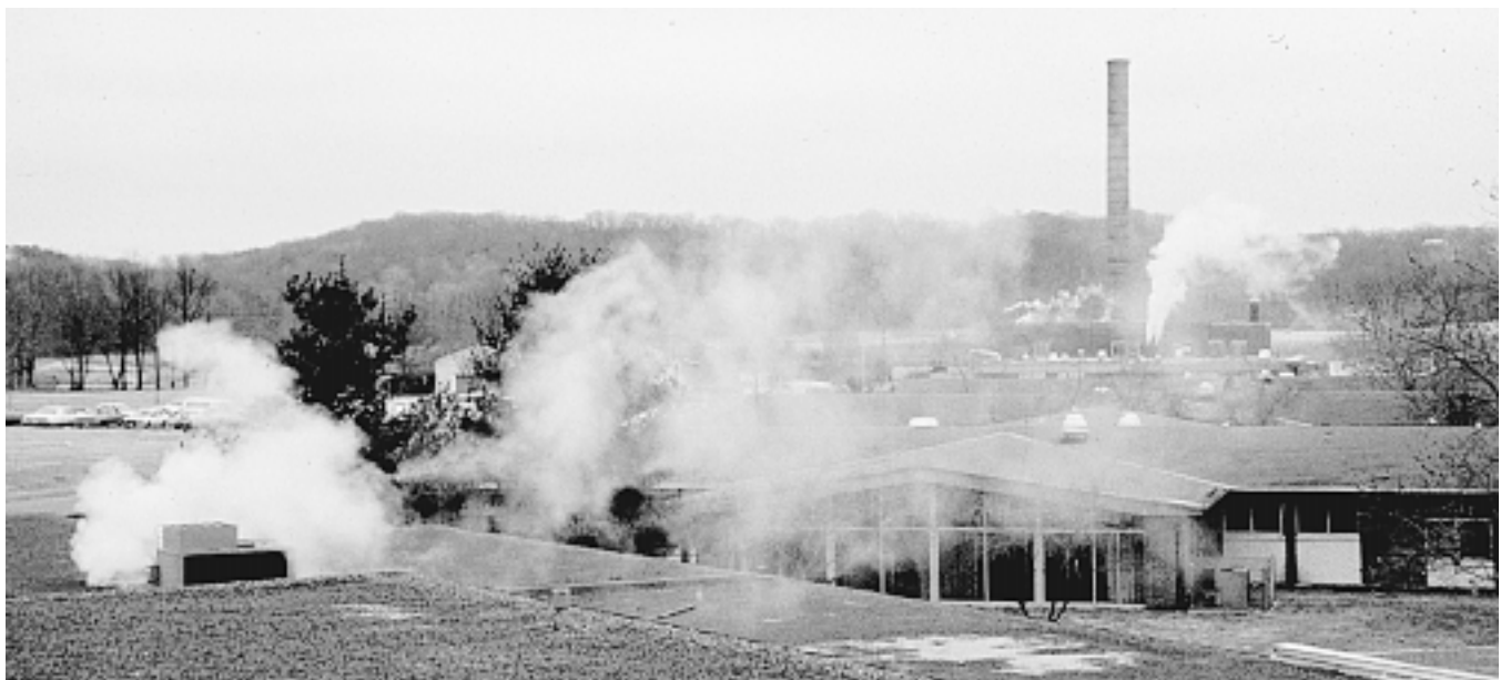
Fig. 1 Major steam leaks This government facility was wasting a lot of taxpayers' money by letting steam escape from the boiler plant and the distribution system.
