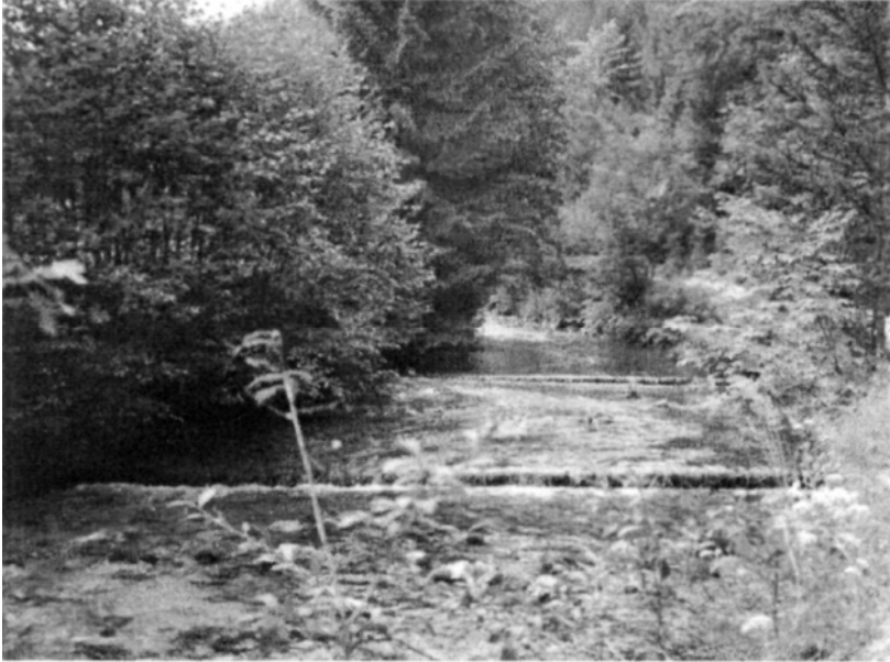
Figure 6.6: Displacement of the axis of flow towards the inner curve, by the use of obliquely positioned logs, which slows down the flow at the outer curve. Freinbach in Steiermark district, Austria.
